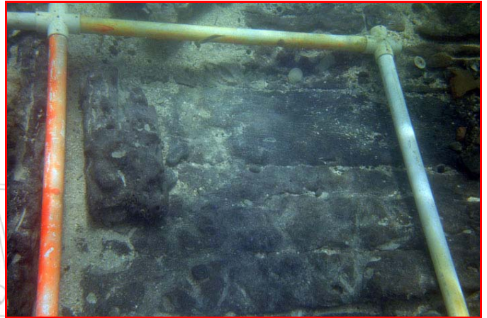
Photograph 27: A cleared section of ceiling planking (© ADMAT).
