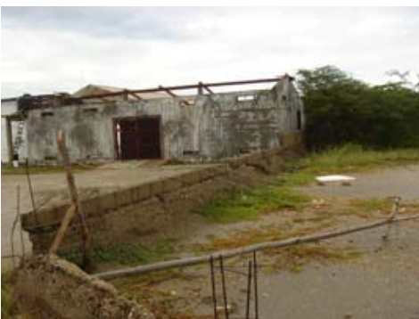
Photograph 21: The roofless building and downed power poles (© ADMAT - Nielsen).
