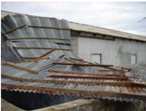
Photograph 20: The blown off roof which landed on some conservation tanks. (© ADMAT - Nielsen).
