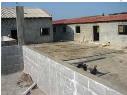
Photograph 13: The Centre dilapidated prior to any work (© ADMAT - Spooner).
